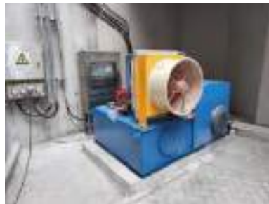
(2) Hydraulic Pump Station
