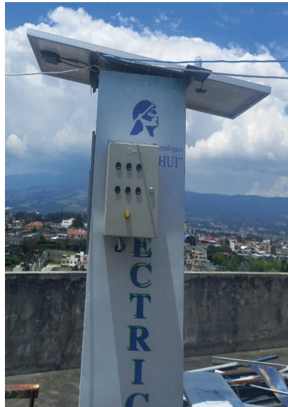
Fig. 4. Test Photovoltaic System.
